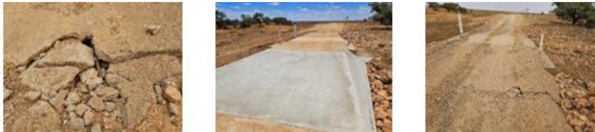
Culvert showing excessive breakage and wear, then completed repairs as required.
