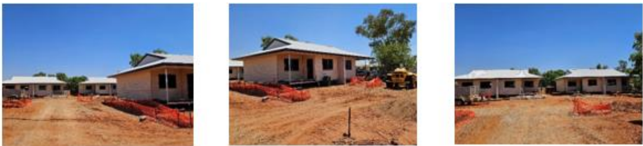
Services, internal works, roof, and walls along with safety compliance: excellent work ethics.
