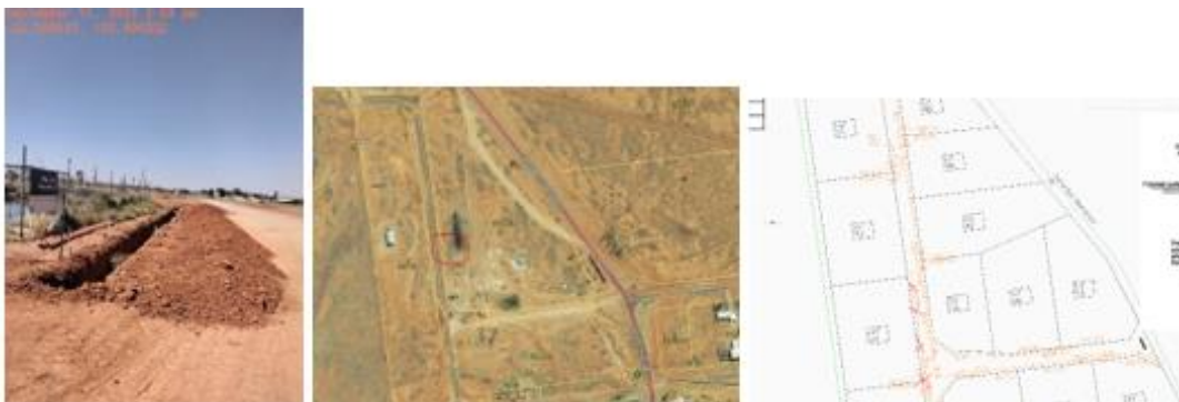
Service trenching by contractors and map showing easement/pad for Transformer and NBN design.
