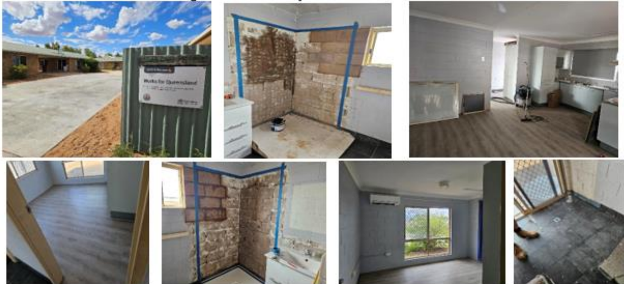
New concrete area design to completion and the second and third units under construction.
