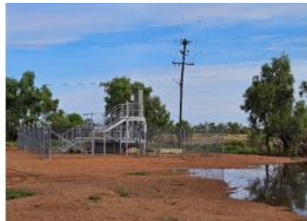
New Pump Station
