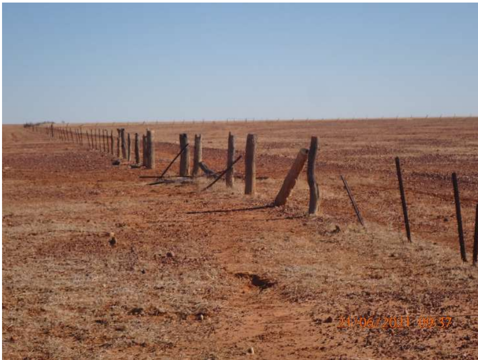
The Pony Club paddock/Kewpie boundary fence is in a sad state, it would be a fair to bad condition with broken/rotten off wood posts and broken wires.
