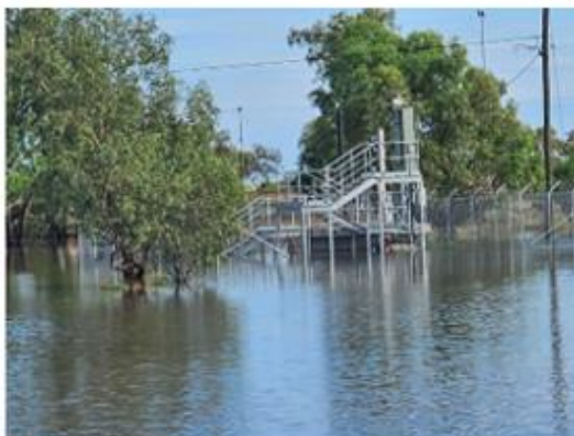
New Pump Station
