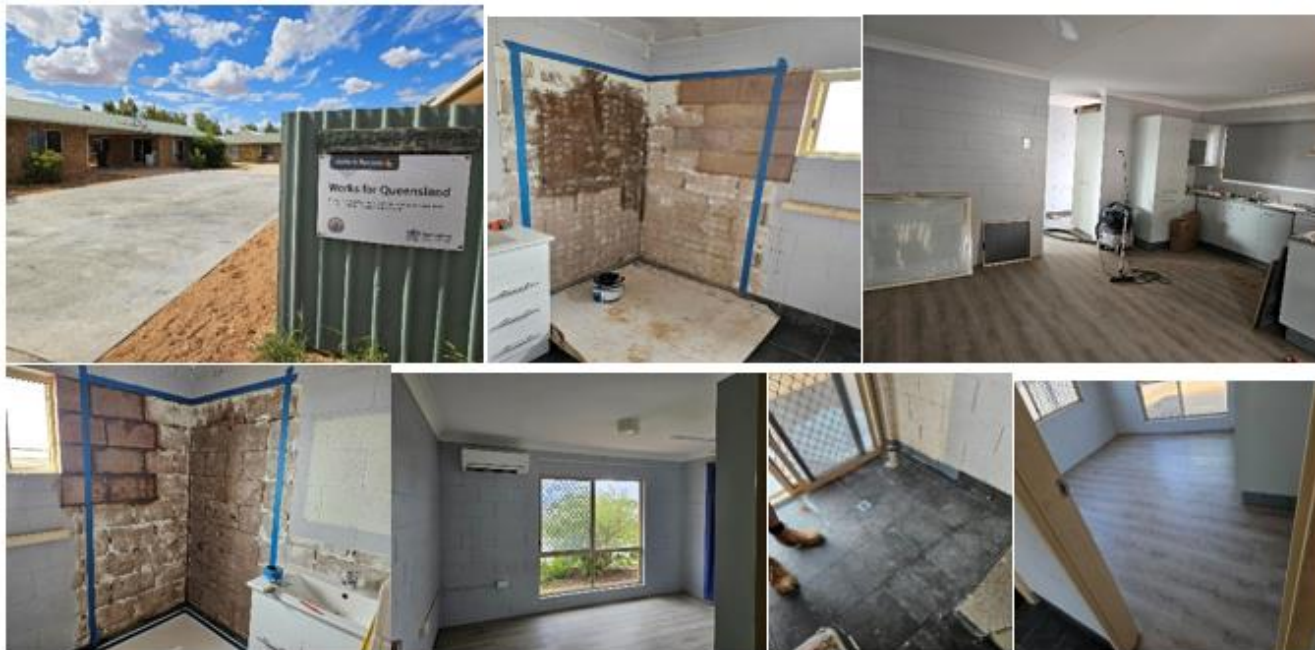
First three units are now complete. Fourth unit almost finished and the fifth unit is now started. All should be complete by April/May 2024.
