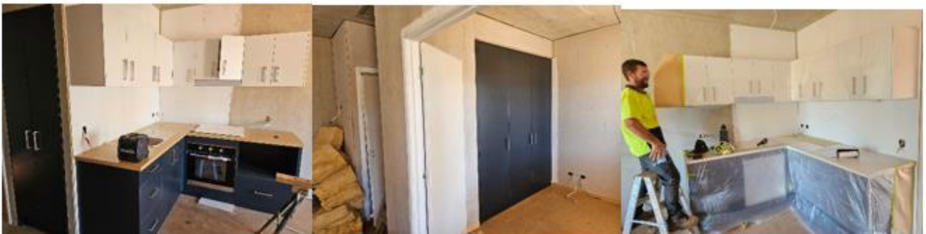
Internal Cupboards have arrived and the shower bases are being put in. Services, internal works, roof and walls are being installed and painted.
