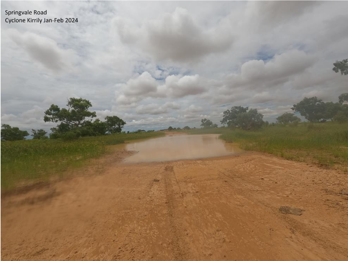
Springvale Road Road damage encountered before emergent works Cyclone Kirrily Jan-Feb 2024
