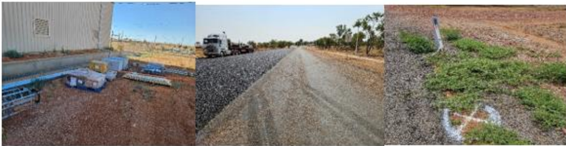
Solar Lights are marked up and services have been identified by Telstra, Lights are ready to be put in.
