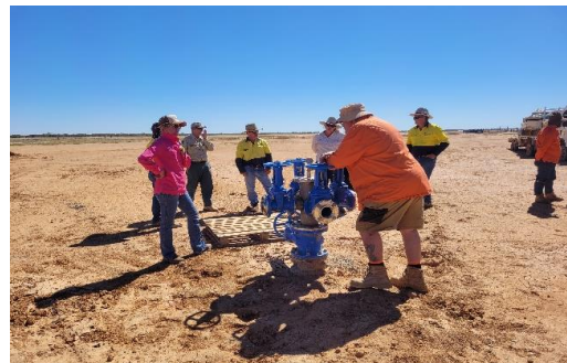
New Mayne Pub Bore.
