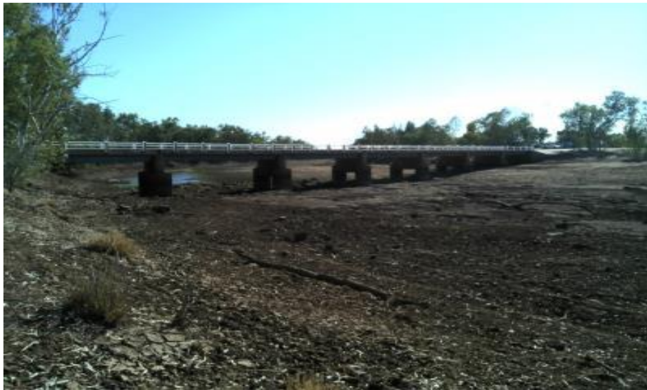
Figure 3.1 Bridge over Burke River forming Kennedy Developmental Road, 100 meter buffer zone required.
